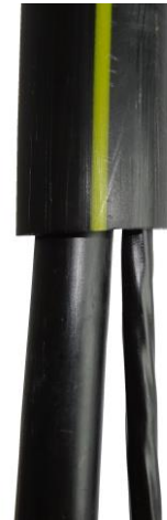
Figure 4. Cables In A 25/20mm Sub-duct.
